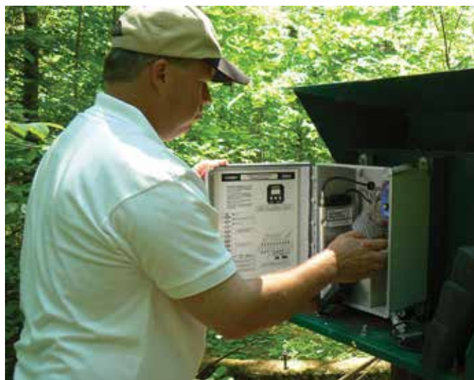
John Bittorf, Water Resources Coordinator, checks the equipment at one of the 10 groundwater monitoring wells.
