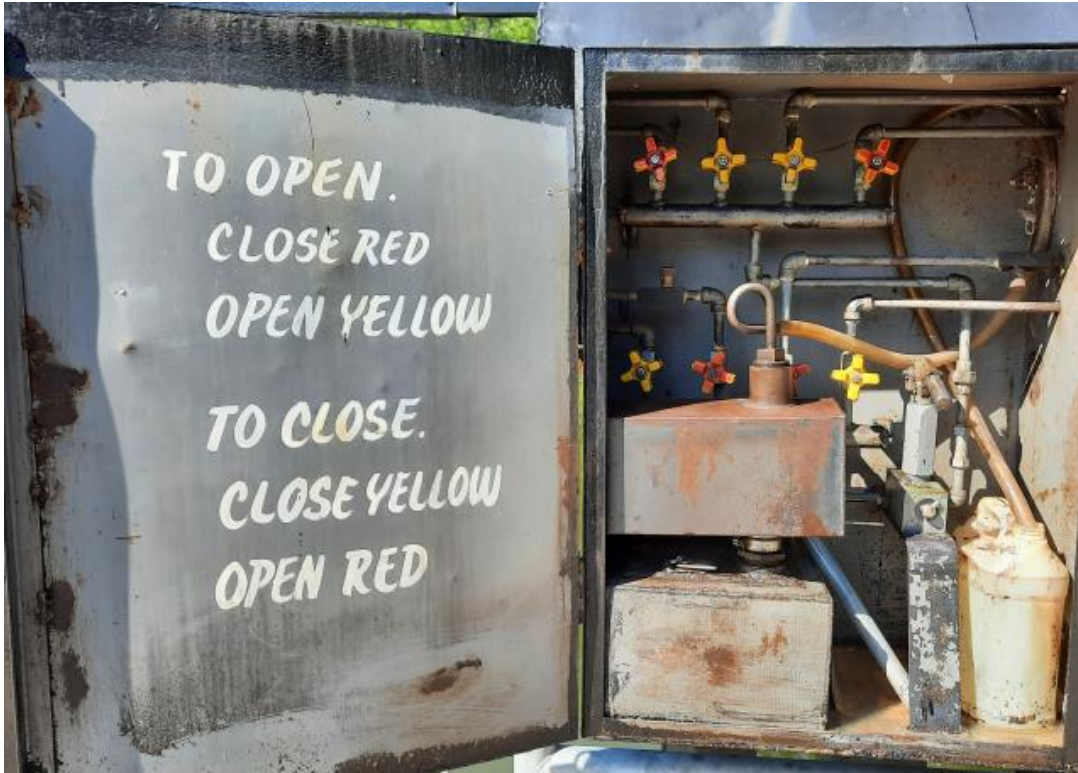
Figure 4 Mill Dam Gate Control Box
