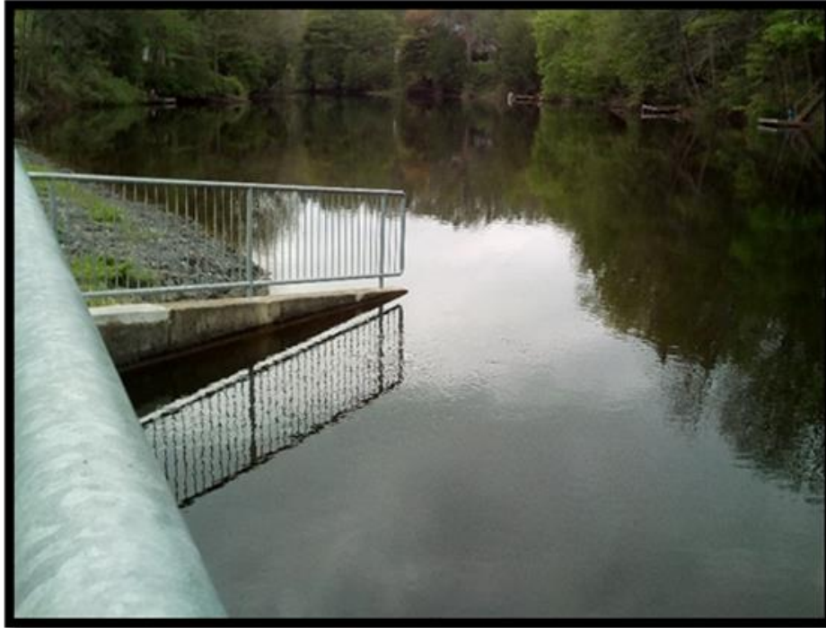
Figure 7 Mill Dam Normal Operating Level (water level +/- 5cm from concrete tip of wing wall)
